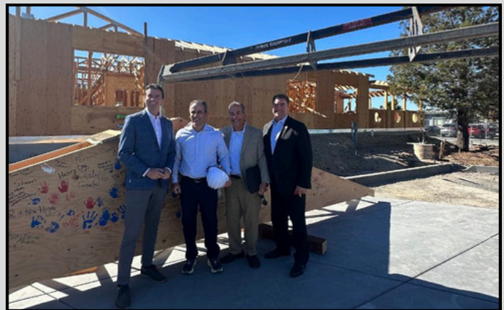
SPEAKING AT THE NORTH BAY CHILDREN'S CENTER AND WATCHING THE INSTALLATION OF THE FINAL ROOF TRUSS OF THE NEW BRIGHT FUTURES CAMPUS
